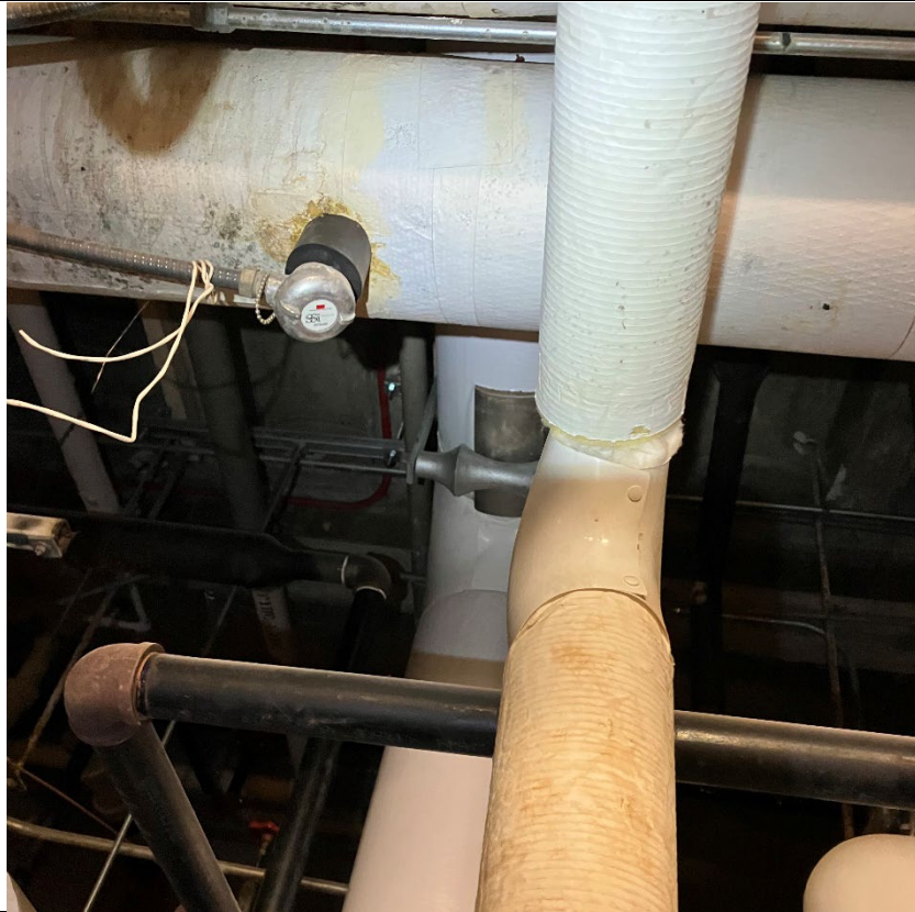
Typical View of Fiberglass Insulation in Mechanical Rooms and Tunnels with PVC Fittings.
