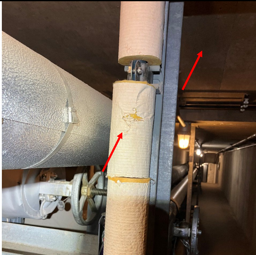
Typical view of Fiberglass Insulation and Metal Covered Foam Glass Insulation in Tunnels.
