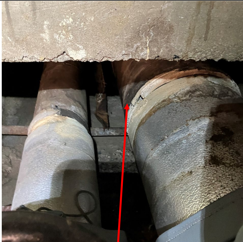
View of Asbestos Pipe Insulation leading into Buried Pipe Chase – 27% Chrysotile Asbestos.
